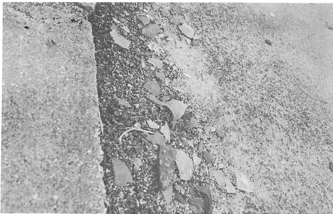
Example of broken glass on the roof surface of the Municipal Water Reservoir
