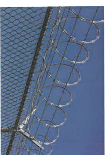
NOT PERMITTED: Wire mesh & razor wire
