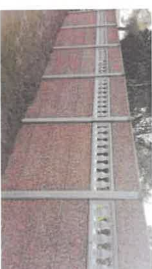
NOT PERMITTED: Vibracrete fence
