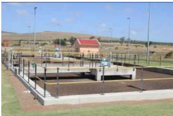
Activated Sludge Reactor
