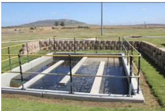
Chlorine Contact Tank
